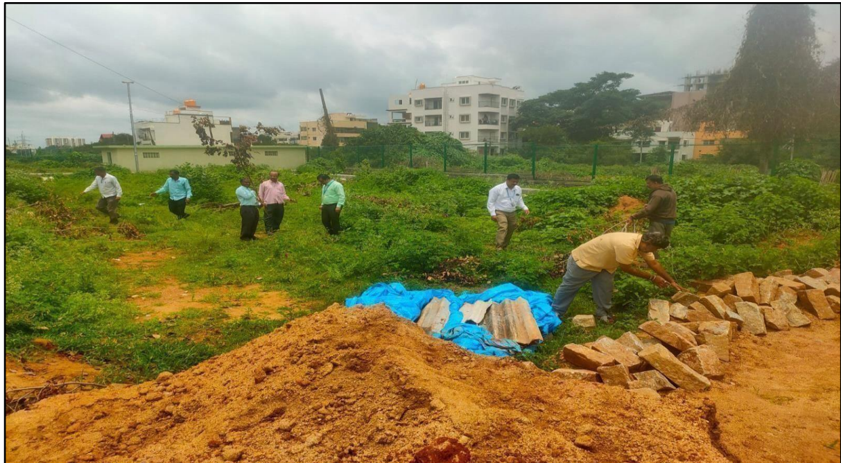
Fig 1: Highlights of cleaning the public ground activity
