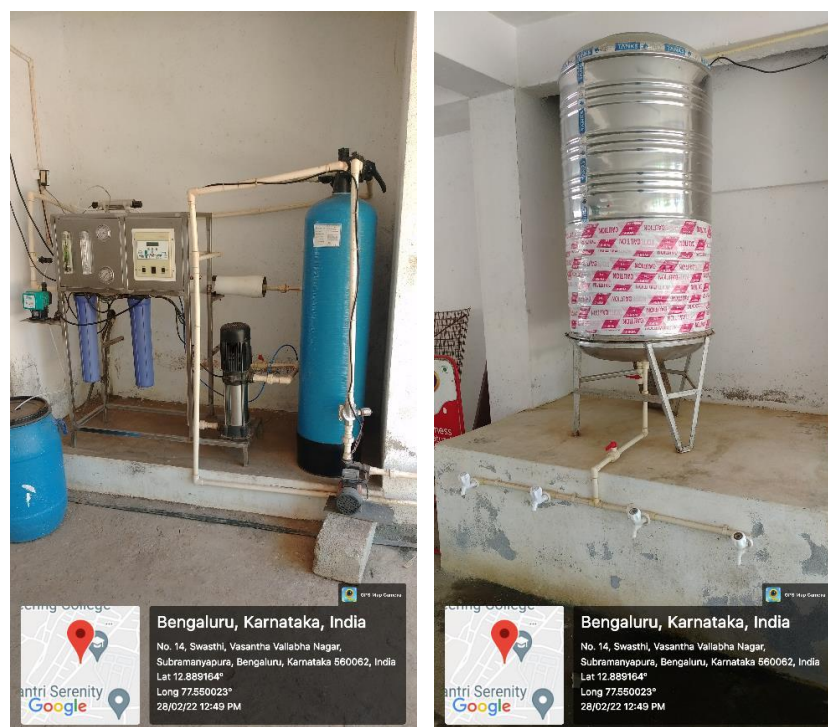
Figure 4-11: RO plant & RO tank
