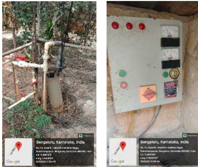
Figure 4-1: Borewell 1 & Control panel (near school block)
