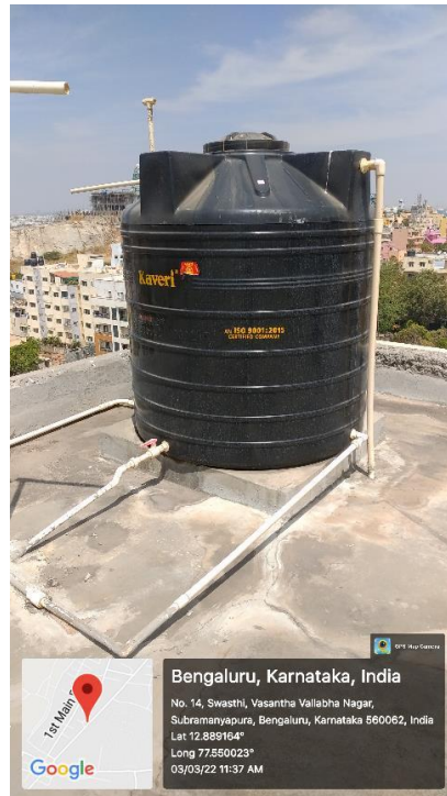
Figure 4-6: 2000 litres PVC overhead tank
