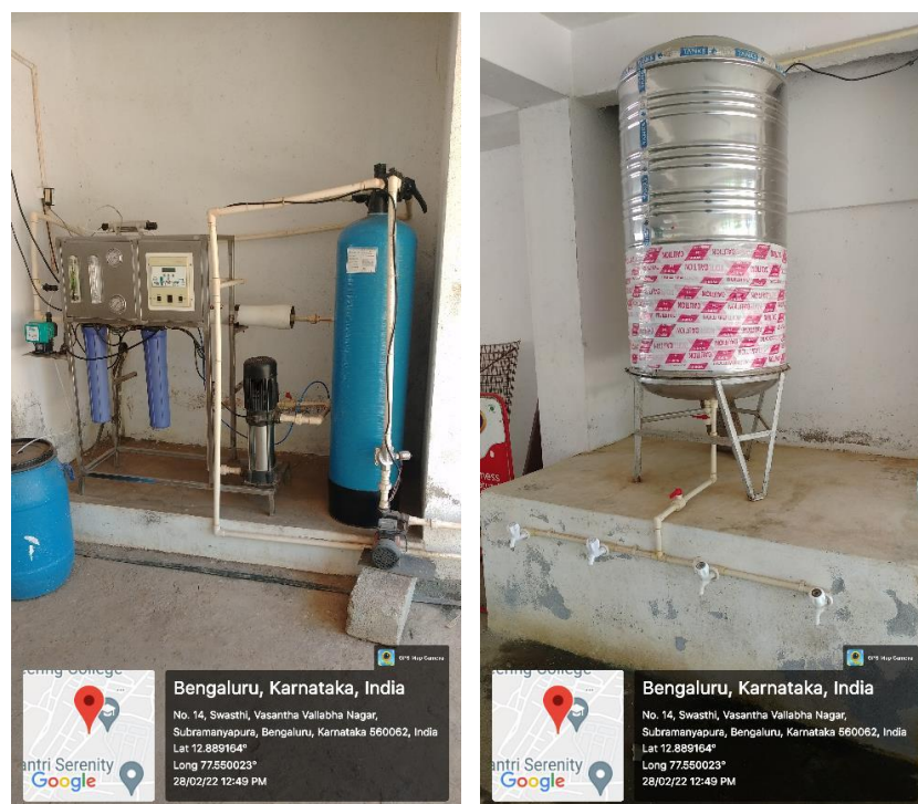
Figure 4-11: RO plant & RO tank
