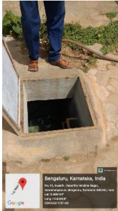
Figure 4-3: Underground sump (near CS/IS block)
