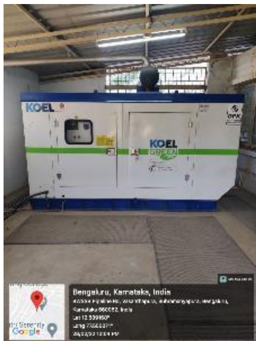
Figure 5-6: Diesel Generator (DG) sets
