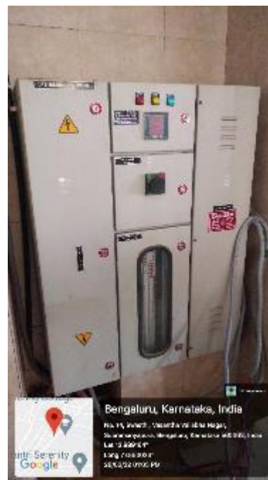
Figure 5-3: Sub-distribution panels for admin block
