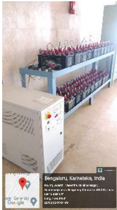
Figure 5-7: UPS in computer Lab - Admin block
