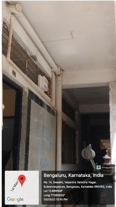
Figure 4-16: Waste water pipeline from rest rooms
