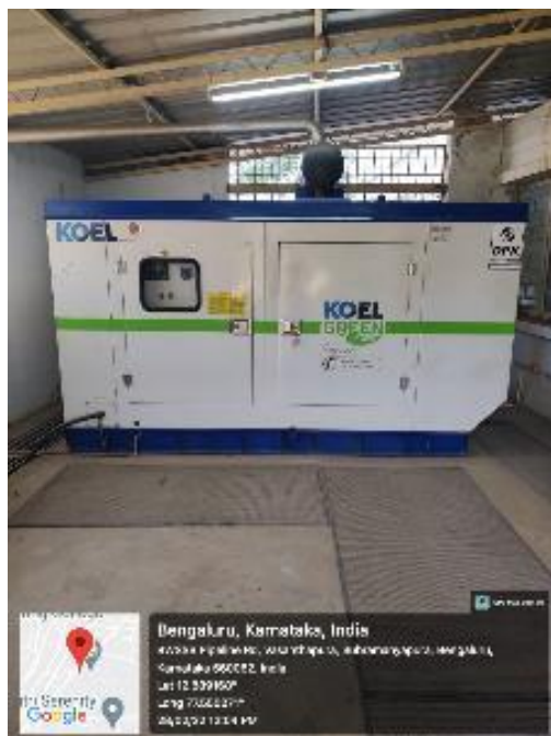
Figure 5-6: Diesel Generator (DG) sets
