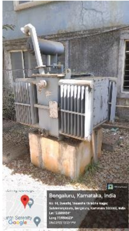
Figure 5-1: Transformer unit Installed in the campus
