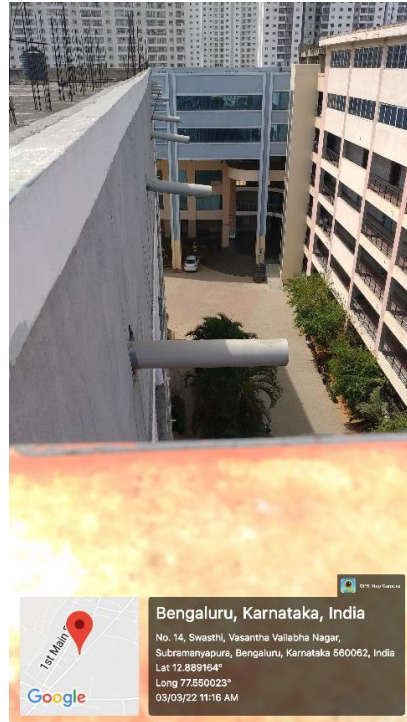
Figure 4-14: Rain water pipes at terrace
