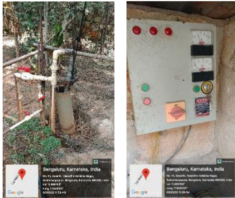
Figure 4-1: Borewell 1 & Control panel (near school block)
