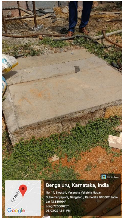
Figure 4-17: Waste water chamber
