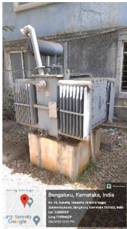
Figure 5-1: Transformer unit Installed in the campus
