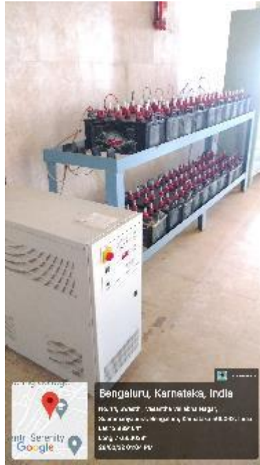
Figure 5-7: UPS in computer Lab - Admin block
