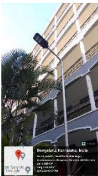
Figure 5-19: Solar LED Street lights with sensors
