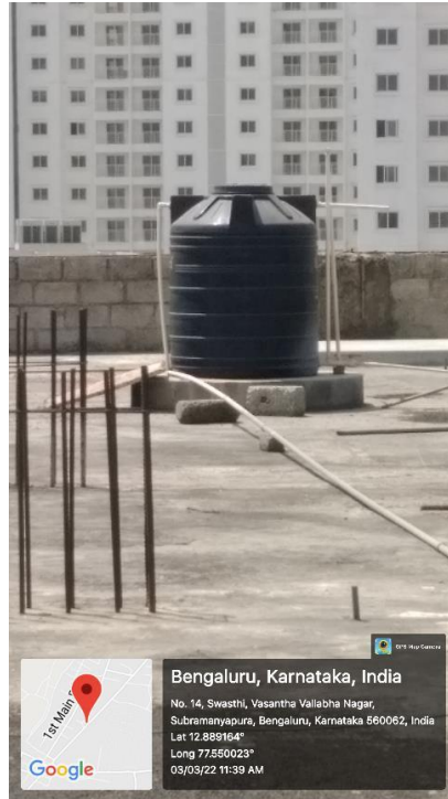
Figure 4-7: 500 litres PVC overhead tank
