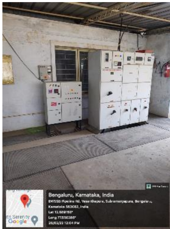
Figure 5-2: Main panel in DG room
